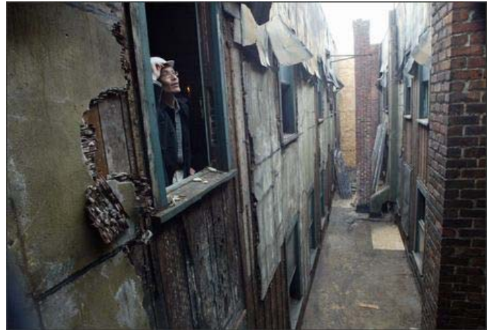
Ron Chew, executive director of the Wing Luke Asian Museum, looks out a newly exposed window well in the East Kong Yick Building.
